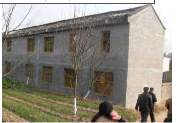
The structural damaged Primary school looks well from the outset.
