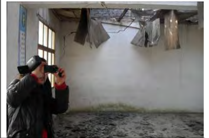
Katherine was taking photo of the structural damage to the roof.
