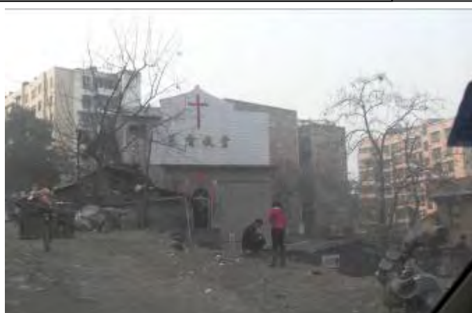
The Ba Chung Church now accommodating 400 is at a very central location but has been classified as unsafe due to earthquake & lack of maintenance. They are still using it anyway.
